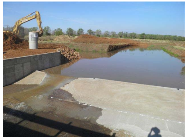
Gauging Station Commissioned
